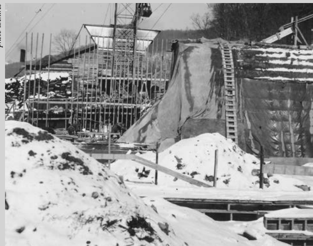
Construction of the Jones Mill Run Dam at Laurel Hill State Park, Somerset County.
