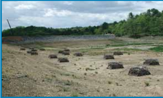
Artificial fish habitats constructed during a drawdown period to rebuild a dam.
