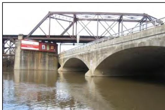
Black River and Western Railroad Bridge No. 77 (Easton Viaduct over 3 rd Street) (Metal Truss Structure)
