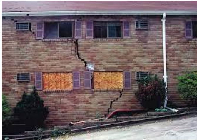
Building damage as a result of subsidence in Pennsylvania. Photo is from a PA DEP Educational Poster for the Mine Subsidence Fund.
