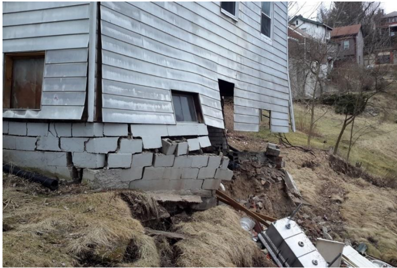
Figure 4.3.9-2 Damage to a Private Home in Pittsburgh
