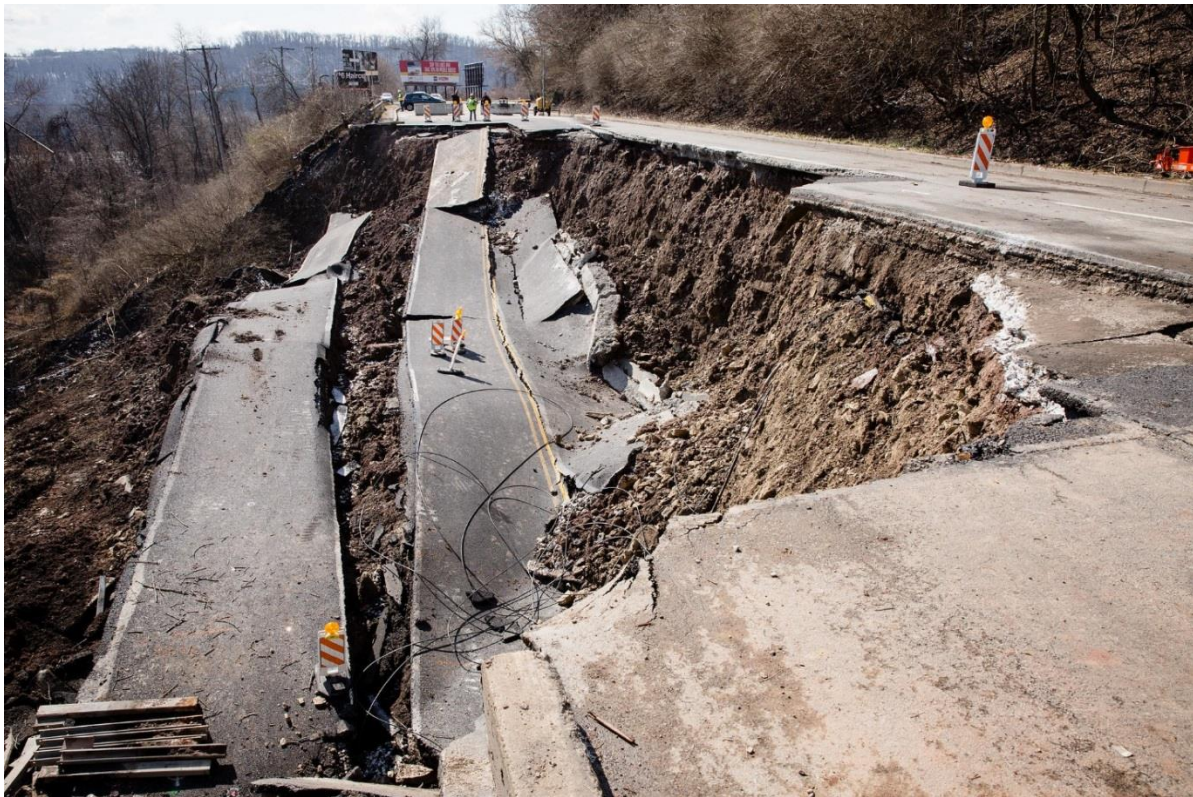
Figure 4.3.9-3 Photo Showing Damage to PA Route 30 due to Landslide Incidents.
