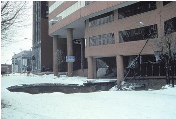
Sinkhole at Corporate Plaza Building in Allentown, Lehigh County, PA in February, 1994 (Photograph by William E. Kochanov . PA DCNR, 2009b).
