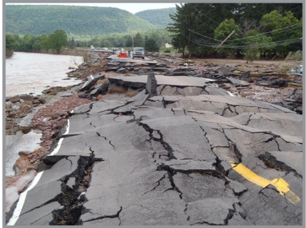
Flood damage to PA 87 in Lycoming County caused by Tropical Storm Lee in September 2011
