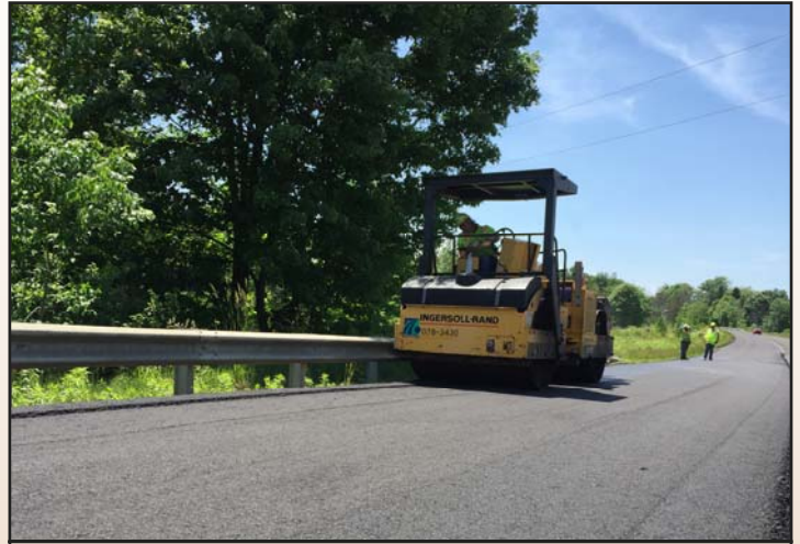
Recycled Asphalt Pavement is rolled and smoothed out during a recent repair project in Venango County.
