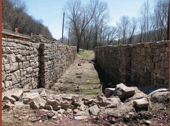
Restored Lock No. 13, April 2008
