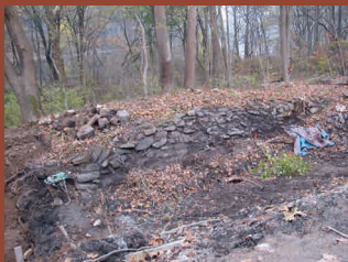
Exposing original stone erosion protection on towpath bank west of lock, November 2007
