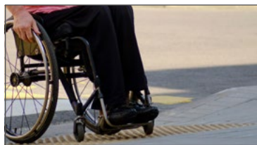
Sidewalks that are not ADA compliant can create barriers for impaired pedestrians.
