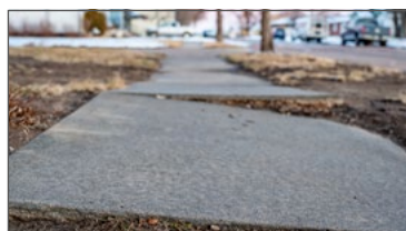
Trip, slip, and fall hazards for pedestrians can result in injury to residents and lawsuits.
