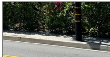
Non-compliant sidewalks can expose pedestrians to conflicts with vehicles in the street.
