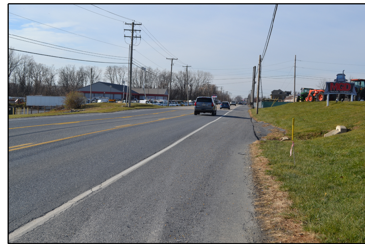
EXISTING SINKHOLE AREA (LOOKING EAST)
