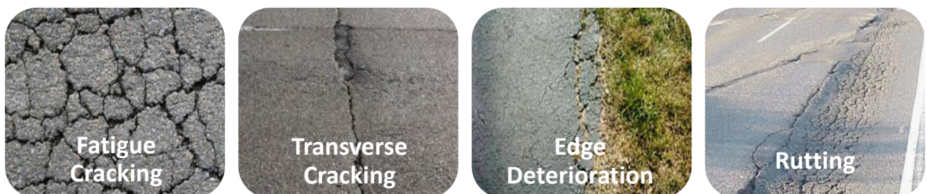
Figure 6: Pavement Damage Examples
