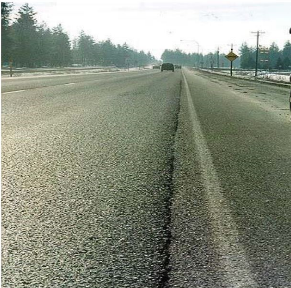
Longitudinal Cracking at the construction joint between the roadway and the shoulder
