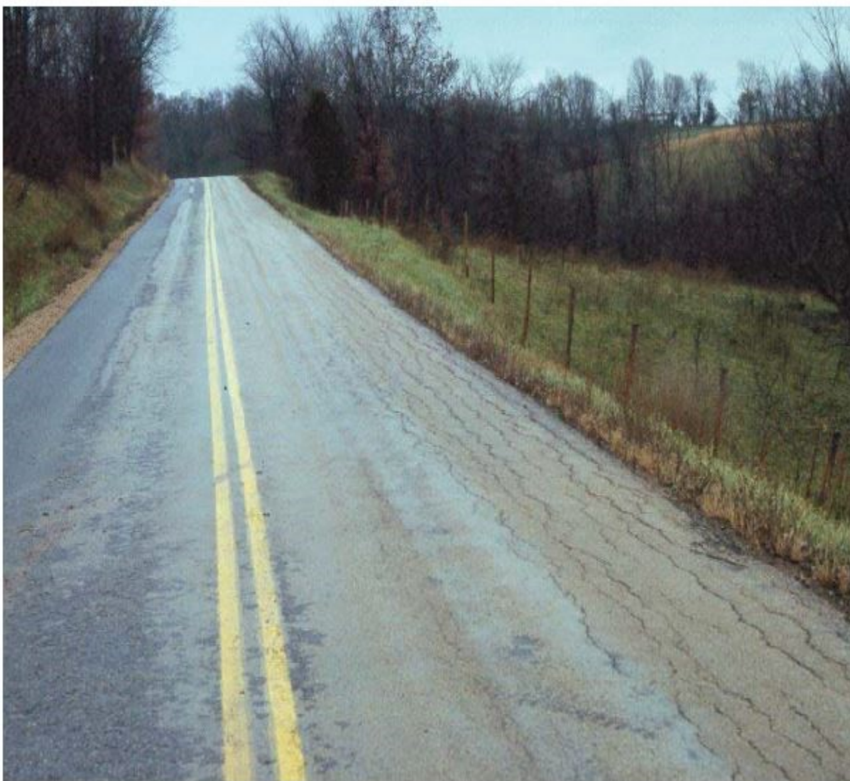
Base Depression with multiple longitudinal cracks in area of right wheel-track and some minor edge breakage
