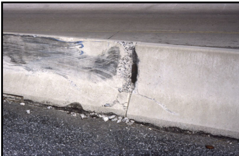
Medium Severity Cracking w/ Spalls
