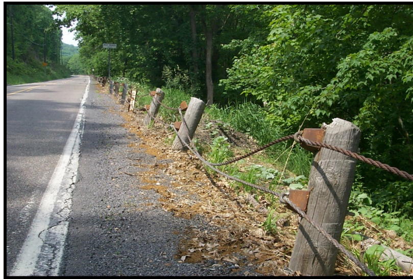
Post Deflection Medium Severity
