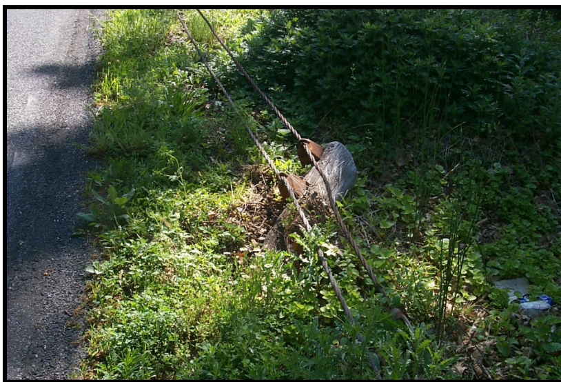
Post Deflection High Severity
