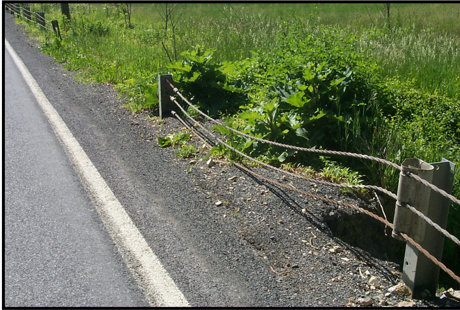
Cable Sag \geq 6'' & \leq 12'' : Medium Severity
