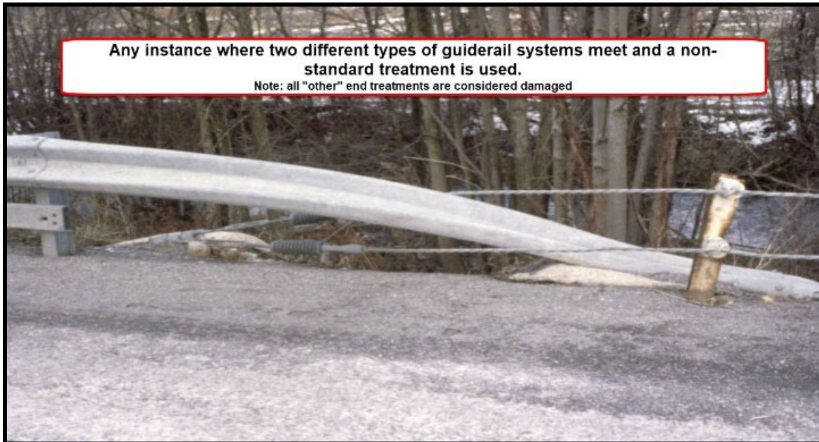
Cable System transition to W-Beam System
