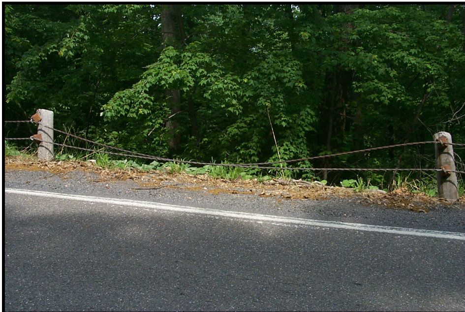
Cable Sag in top cable > 12'' , bottom cable none: High Severity
