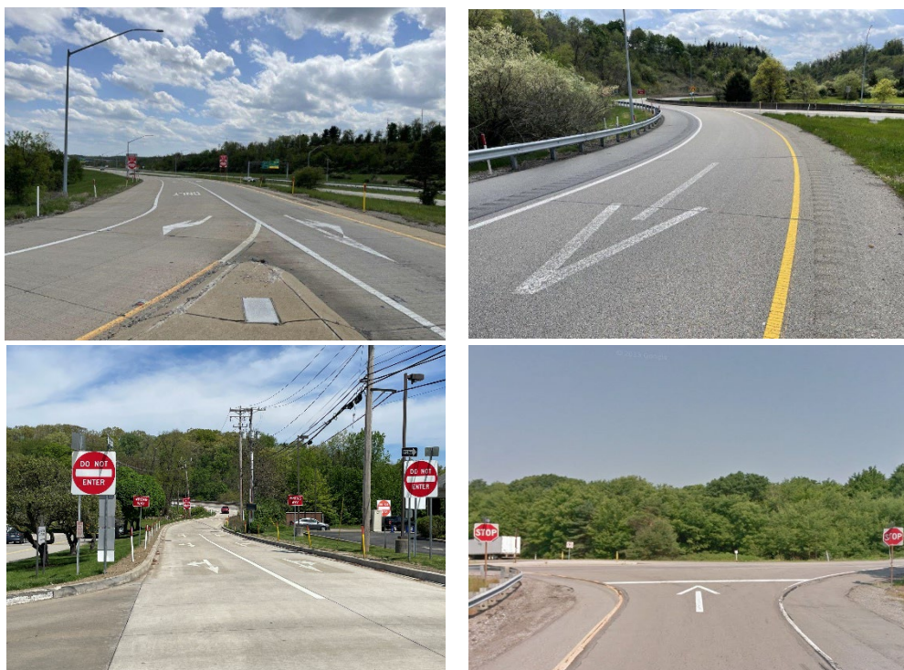
Figure 5.7.16–4: Examples of Upgraded Pavement Markings
