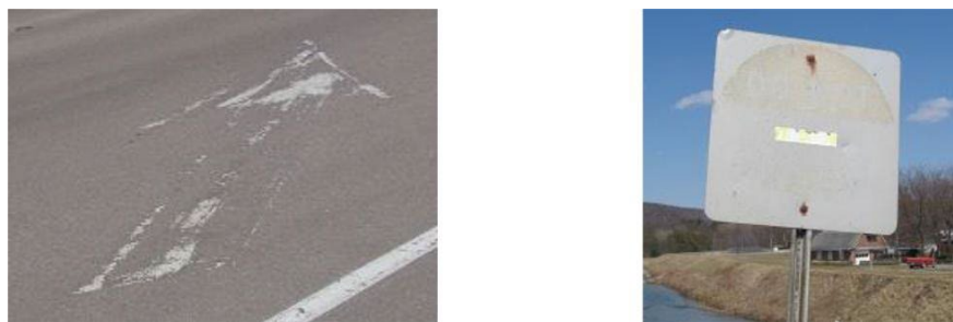
Figure 5.7.16–1: Examples of Poorly Maintained Pavement Marking and Signage
