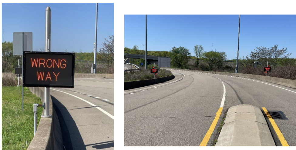
Figure 5.7.16–5: Example of LED-Enhanced Wrong-Way Signage
