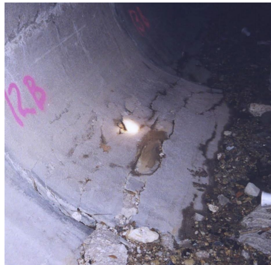
PHOTO NO. 3, Example of Radial Tension Cracks
