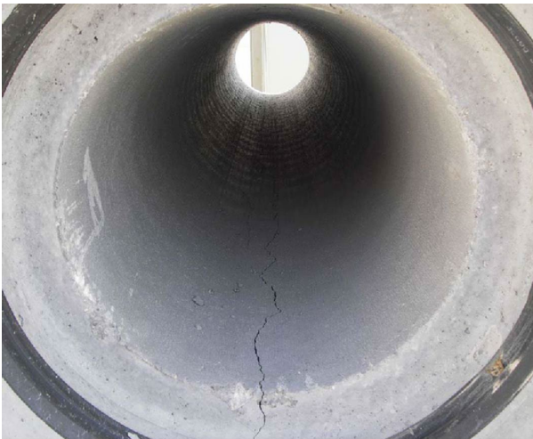
PHOTO NO. 1, Example of Flexural Crack
