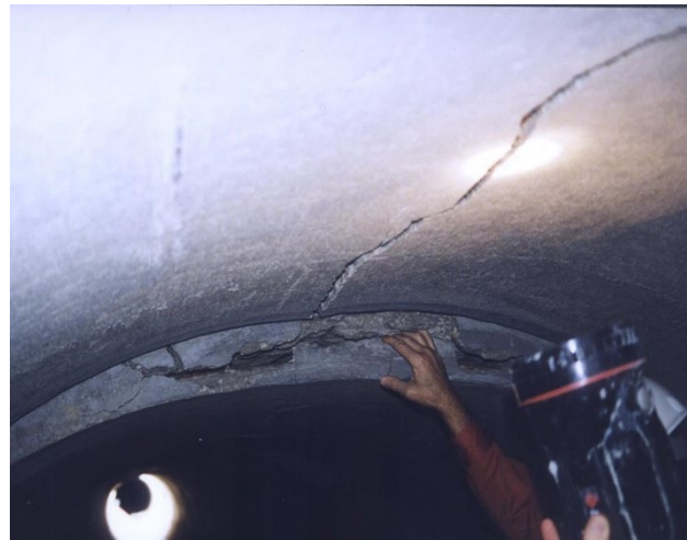
PHOTO NO. 2, Example of Shear Crack
