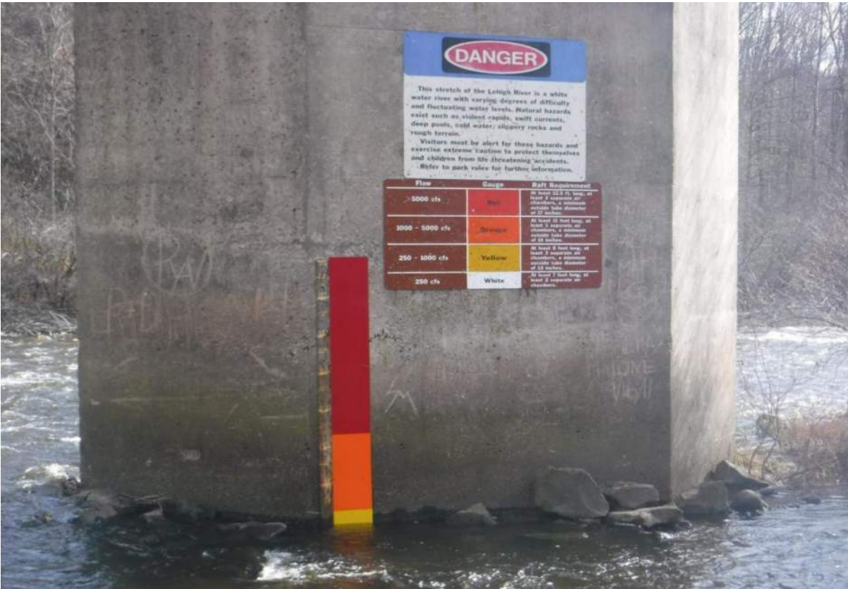
River gauge and raft requirements posted on the eastbound I-80 Lehigh River bridge pier
