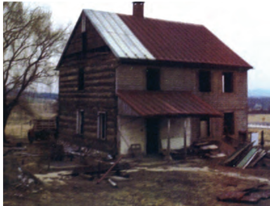
The farmhouse during its demolition in 1971. The log construction of the house was visible beneath the wooden siding. (Photograph courtesy of Fayne Hartman)
