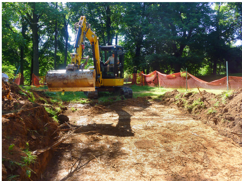
A backhoe strips plow zone soils from a portion of SRT-4 in July 2018.
