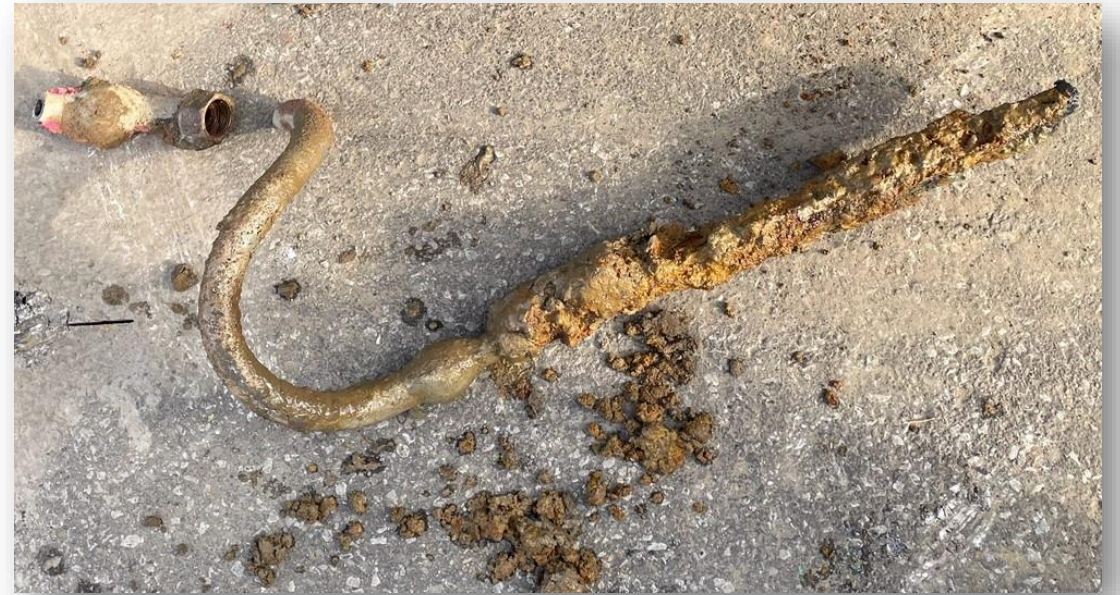
Example lead gooseneck and corroded lead service line Erie City Water Authority - City of Erie, Erie County
